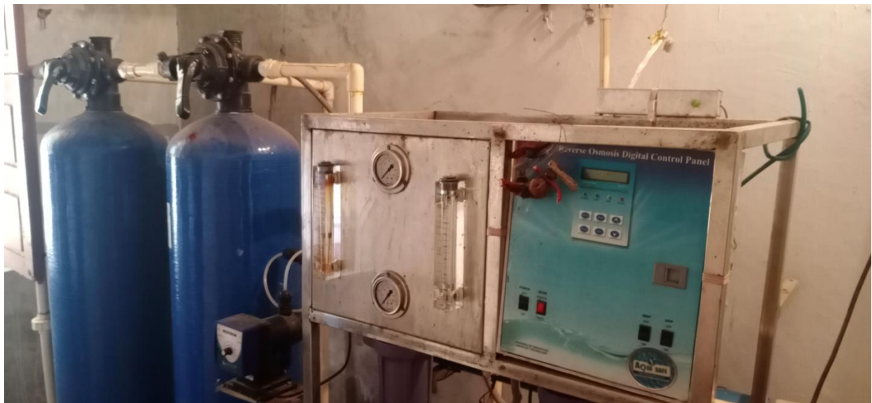
RO drinking water facility in college
